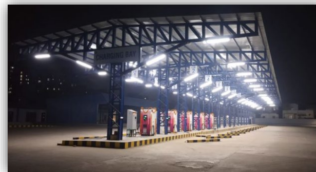
Charging Equipment Protection
